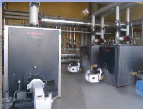
Gas boiler-house for the Daugavpils City Central Market Pavilion "Gallery" Year 2002.
